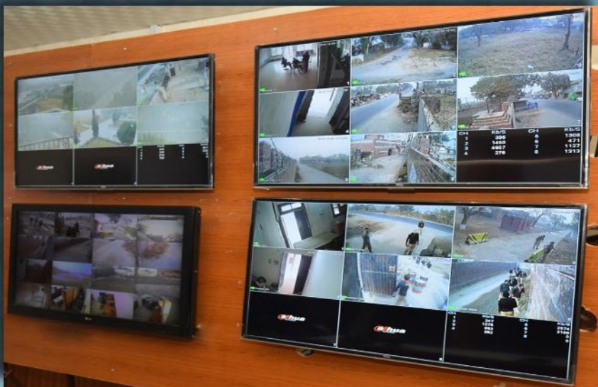
"Control Room" Keeping in view the latest technology PTC Sihala is using the latest and up to the mark CCTV Cameras for its security, as well as panic alert system for prevention of unwanted entry
