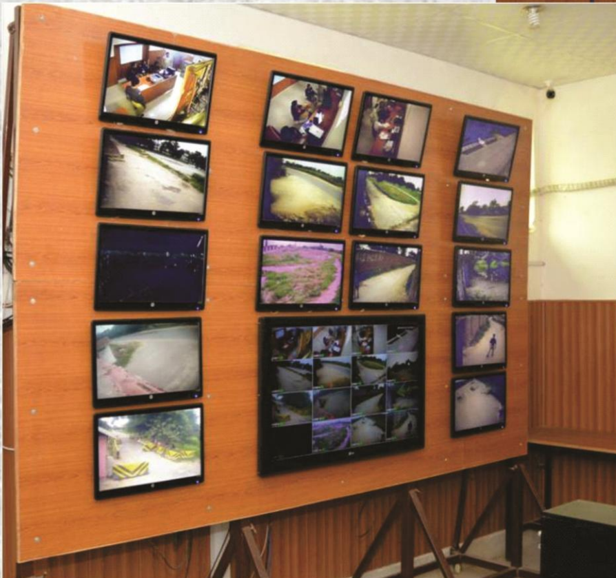
State-of-the-art Control Room
